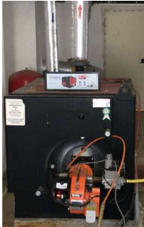
Figure 7: The natural gas heating system used in the lodgment apartments
